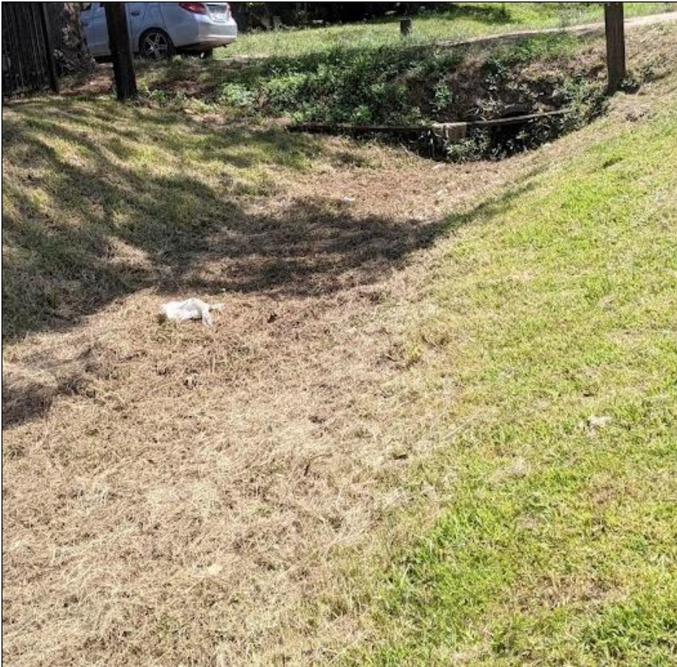
Figure 12. Picture of open drainage ditch in Northeast Houston with culvert non-functional.
