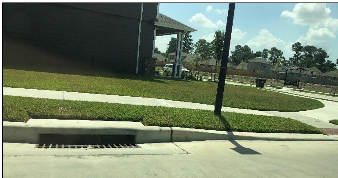
Figure 20. A drainage inlet in the old section of Northwood Manor (top) vs. a drainage inlet in a new development of Northwood Manor (bottom).
