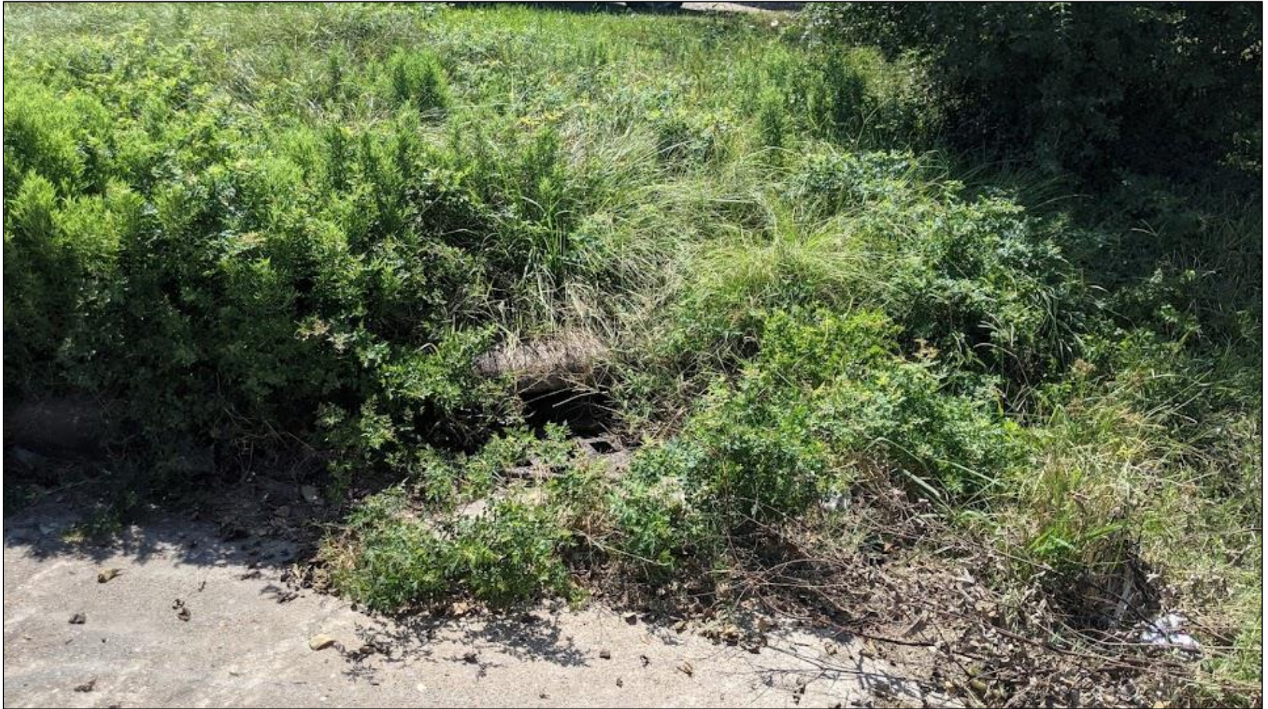
Figure 19. A drainage inlet on an uninhabited property in Northwood Manor which is almost completely covered by overgrown plants and debris.
