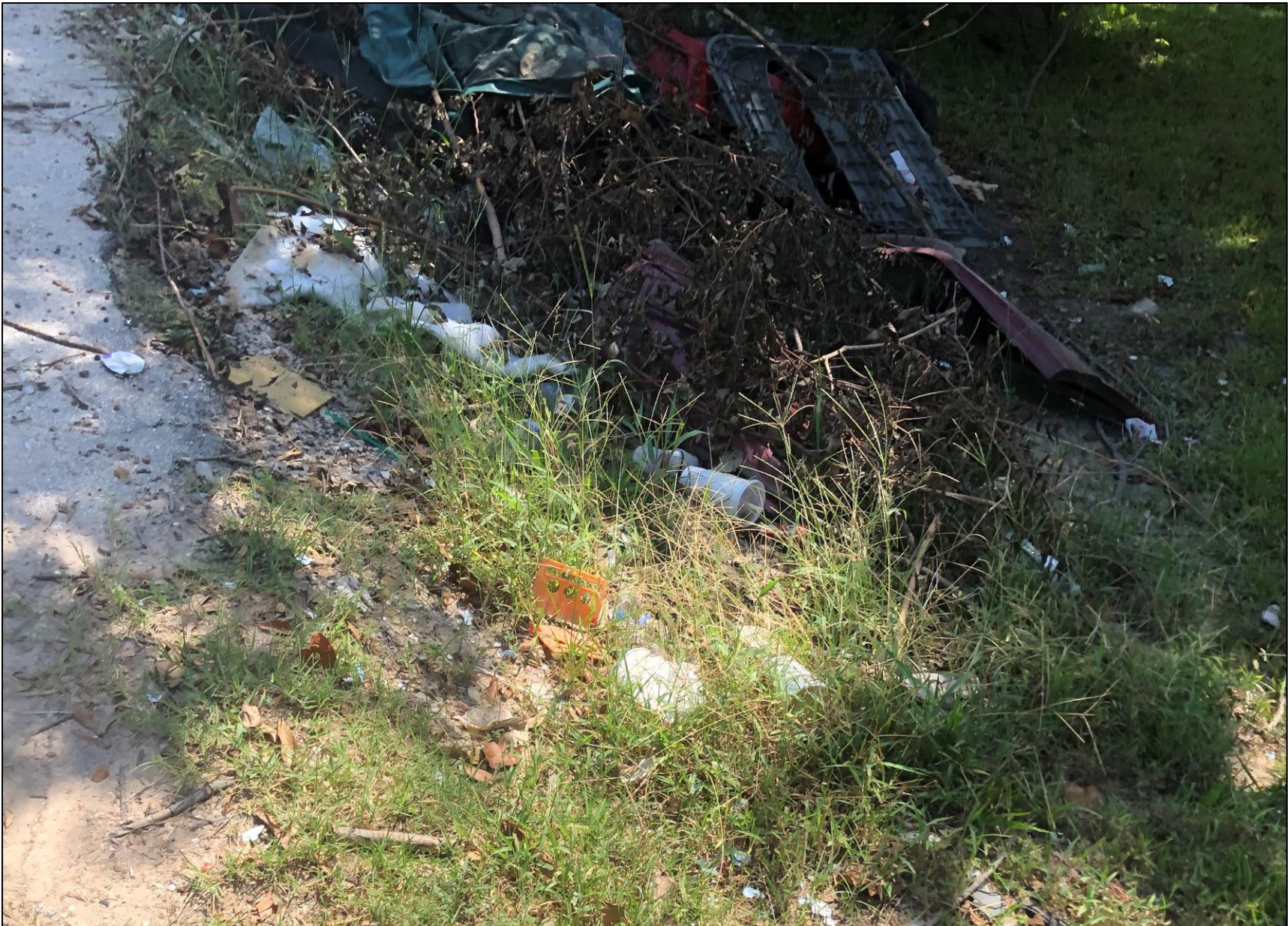
Figure 16. Open drainage ditch in Northwood Manor with trash piling up and obstructing drainage.
