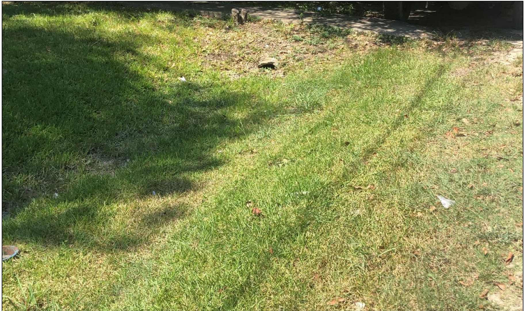
Figure 13. Picture of open drainage ditch in Northeast Houston with culvert non-functional.
