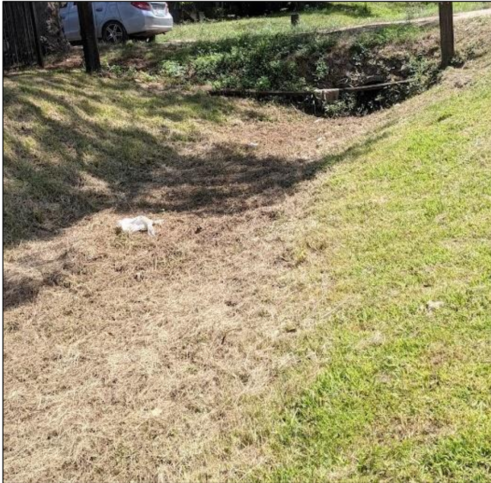
Figure 12. Picture of open drainage ditch in Northeast Houston with culvert non-functional. Photo by Sarah Swackhamer.
