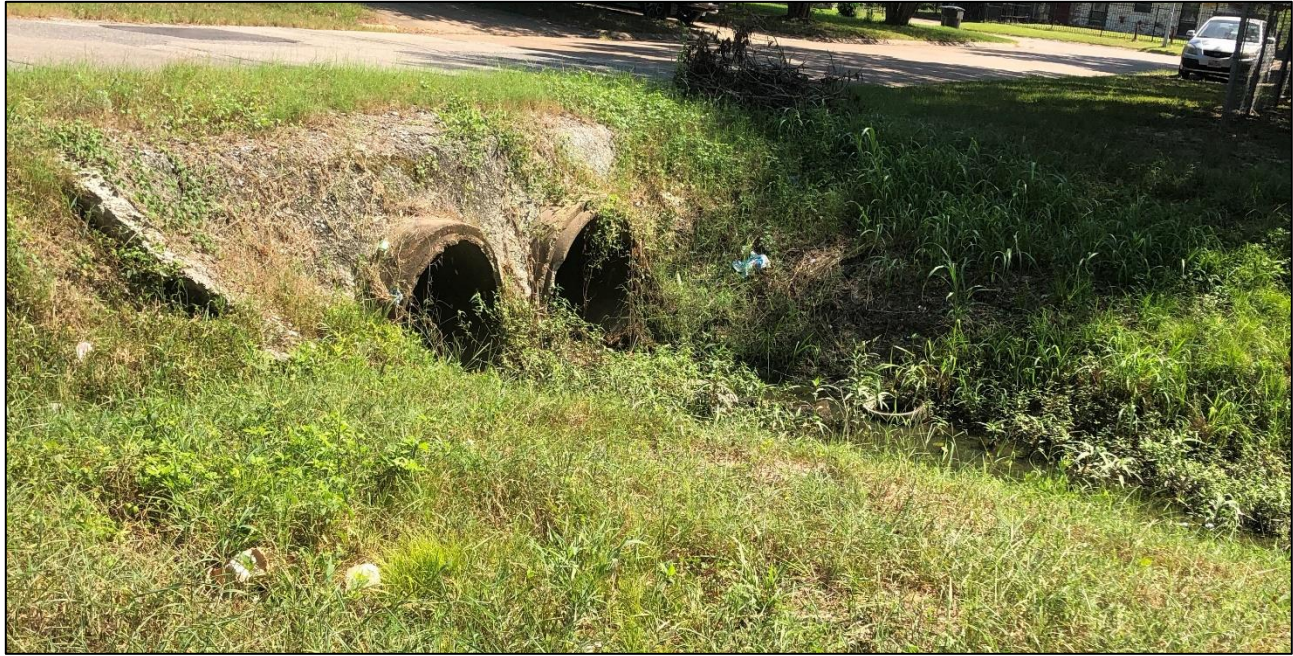
Figure 18. Inlets of the Harris County P125 drainage ditch. Pictures from Camille Chenevert.
